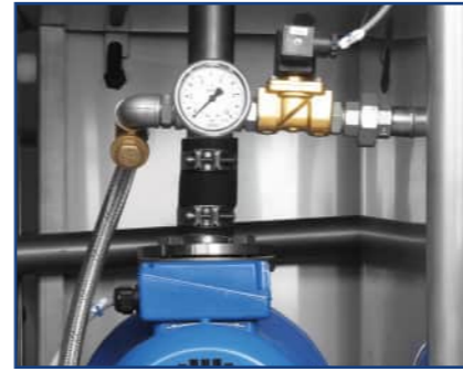
Image 08 Pressure gauge for pressure testing - simple function check
